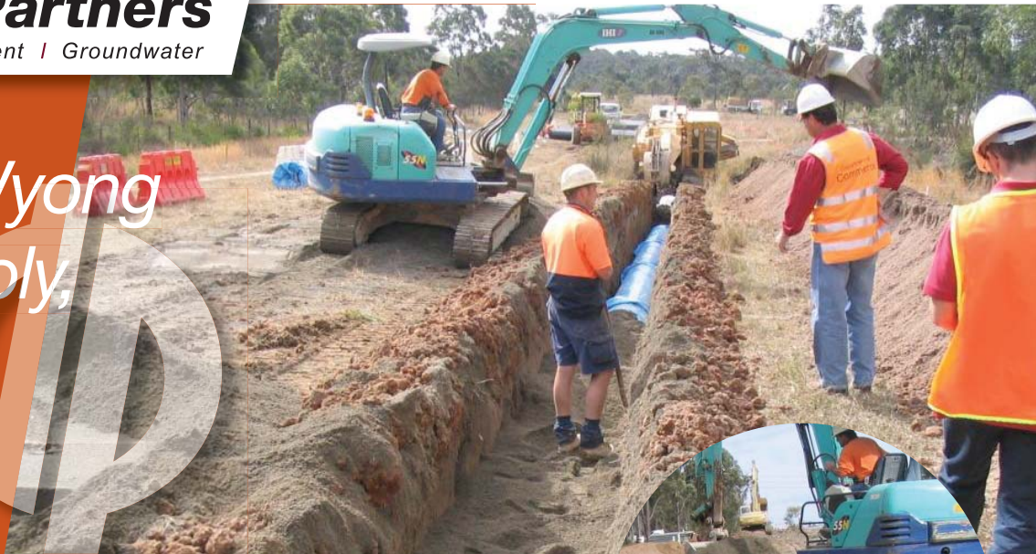
Stage 3 construction of pipeline from Morisset to Warnervale – image courtesy of Worley Parsons
