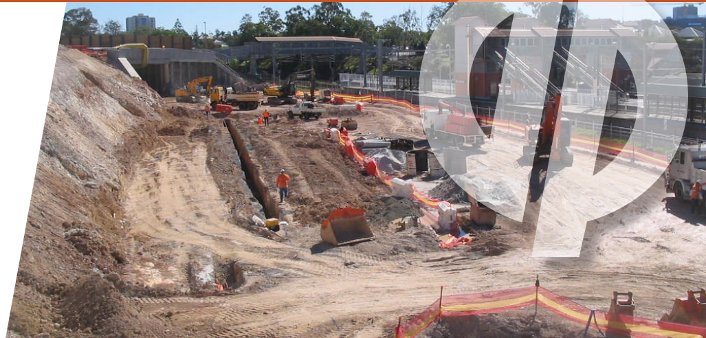
The 1.5 kilometre Boggo Road Busway provides crucial public transport access connecting to the existing rail station.
